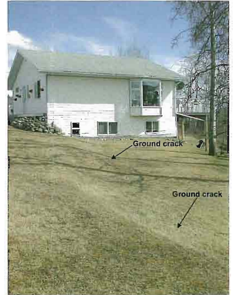
Photo 15: View south east at 195. Note ground depression/fresh cracking that can be traced to north west side of house and crack in north west foundation wall. This represents the likely new main scarp of a deep-seated landslide into Bulkley River.
