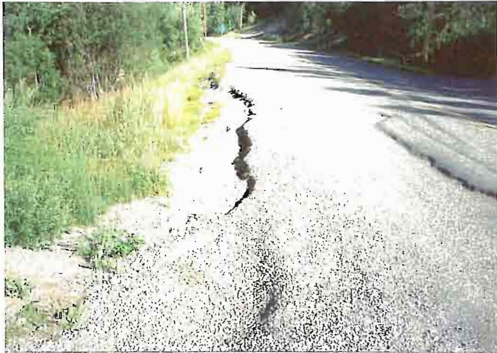
Photo 11: MoT photo (ca. 1989), looking north at fill failure on Lower Viewmount Road just north of driveway access for 1037.
