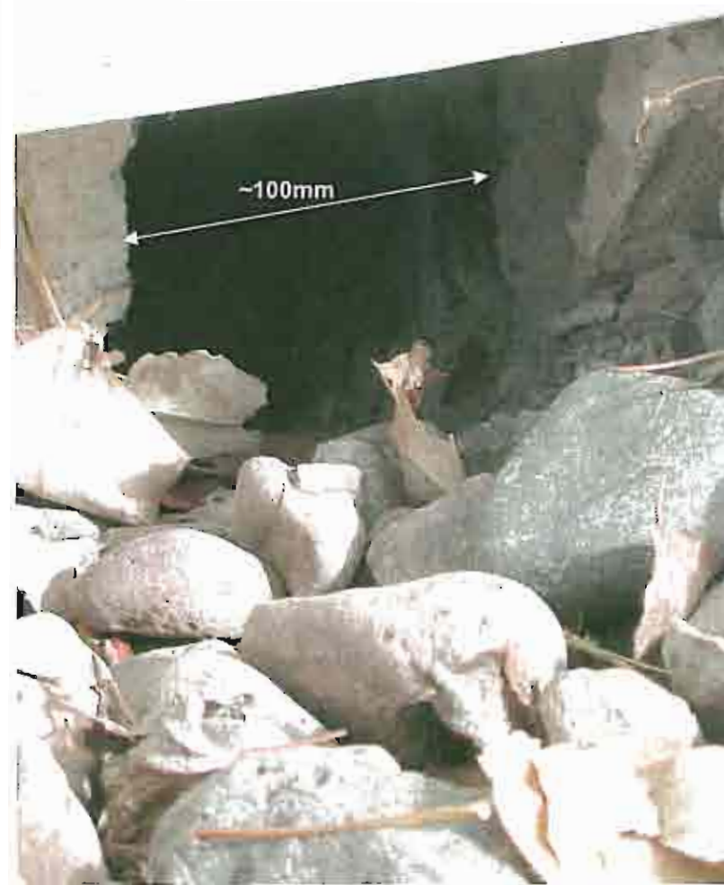
Photo 17: An approximately 100 mm wide crack in basement concrete wall on north west side of 195.
