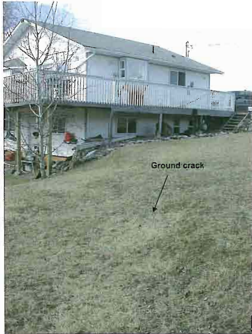
Photo 16: View north at 195 along ground depression/fresh cracking that can be traced to south east foundation wall of house.
