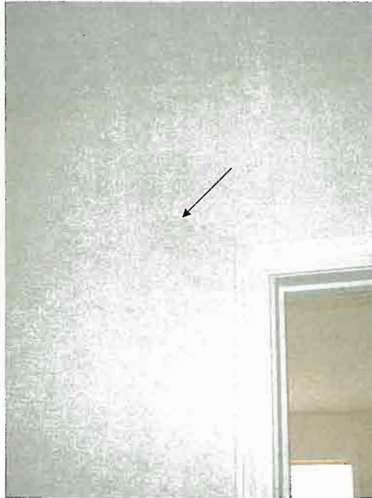
Photo 21: Typical cracking in gyproc on the basement level of 195.
