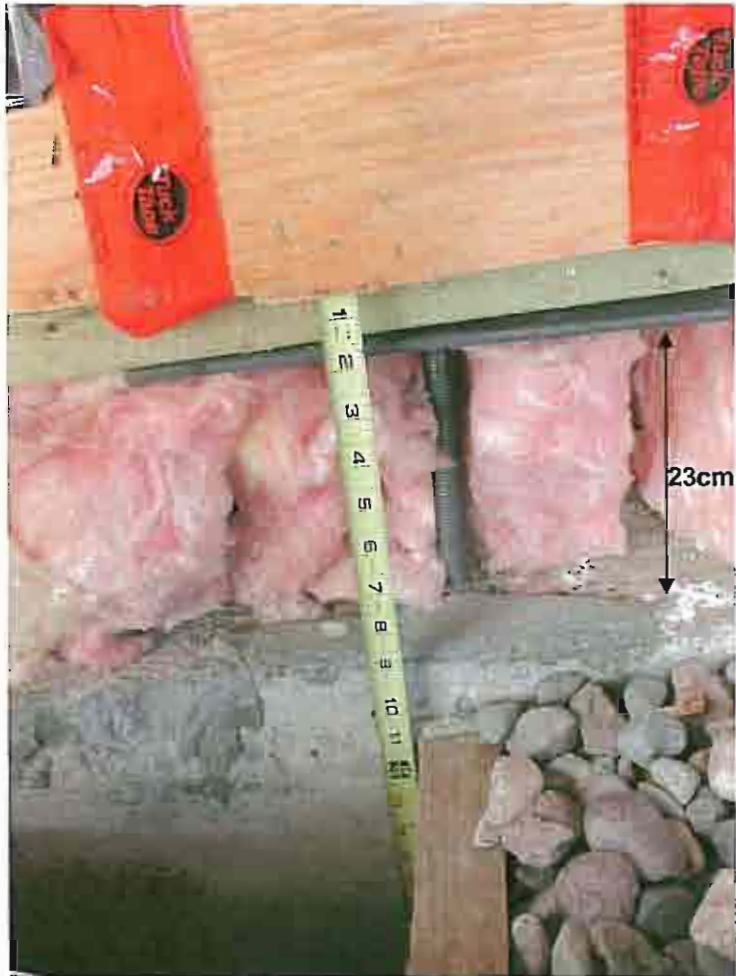
Photo 19: Close up view of a foundation jack on south west side of 195. Note total vertical displacement of approximately 23 cm (9inches).
