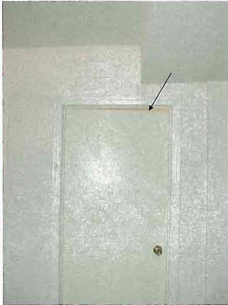
Photo 20 Typical distorted interior door frame on the basement level of 195.
