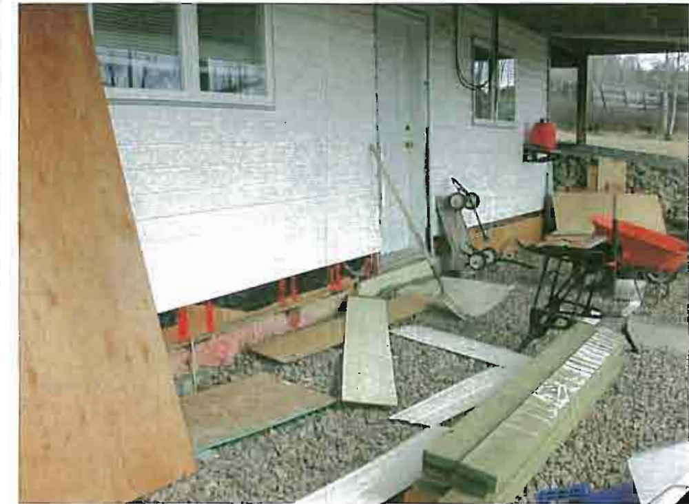
Photo 18: Exposed jacking system on down slope (south west) side of 195.
