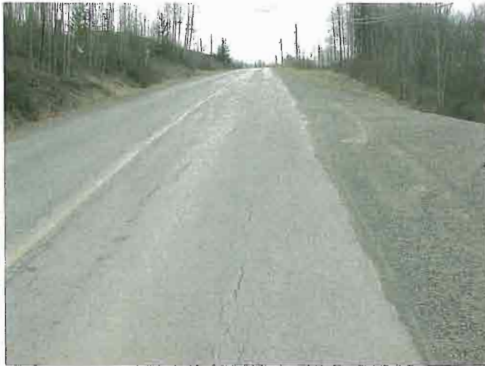
Photo 5: View south at pavement deformation on Lower Viewmount Road due to a fill failure in the vicinity of the driveway for 1037.
