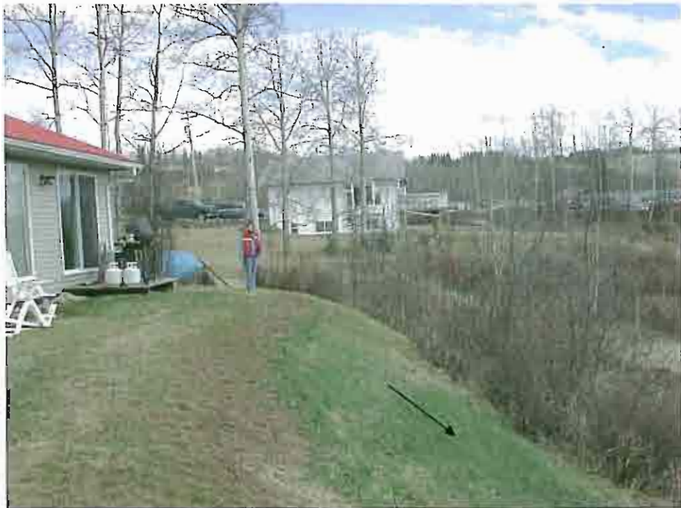
Photo 27: Looking south east along main scarp of landslide behind 265 towards 195. Note that community water line and septic line crosses this scarp area.
