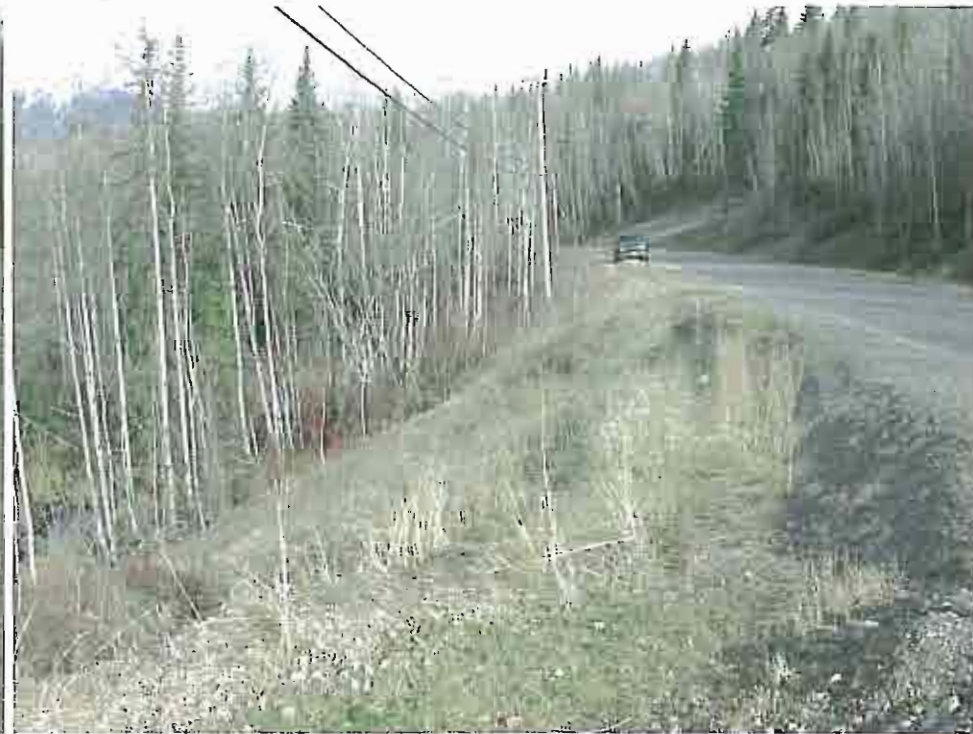
Photo 6: View north at fill failure on Lower Viewmount Road, just north of driveway entrance for 1037.
