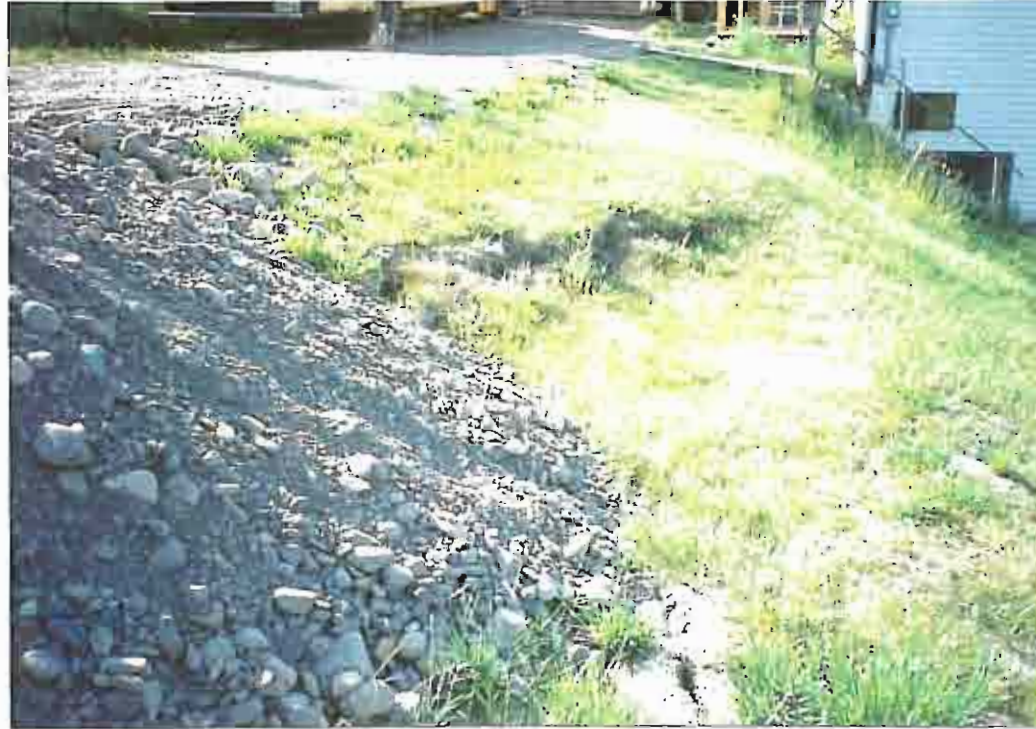
Photo 12: MoT photo (ca. 1989), looking south west at ground cracking in fill below driveway of 1037.
