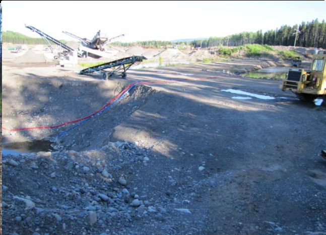
Looking south at wash plant &amp; pond arrangement
