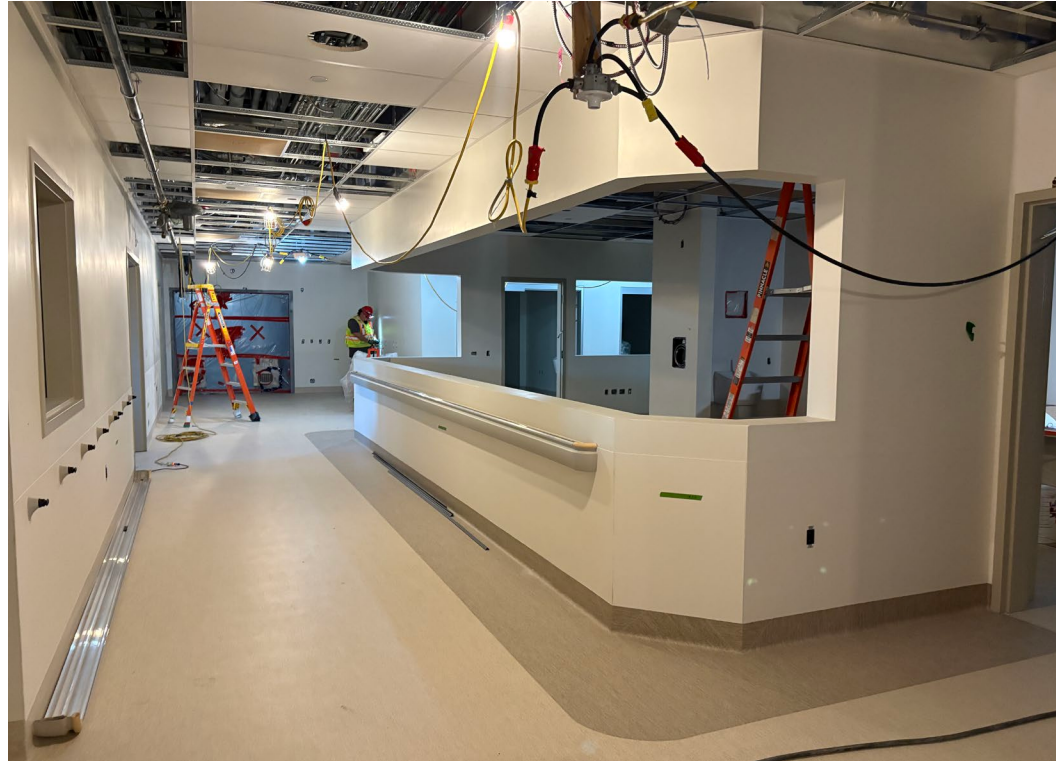
Emergency Department Care Station
